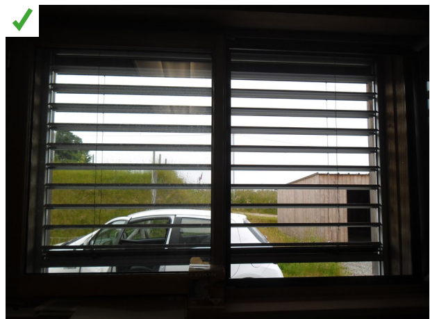
Brise-soleil orientable - Façade Est. ©AQC
